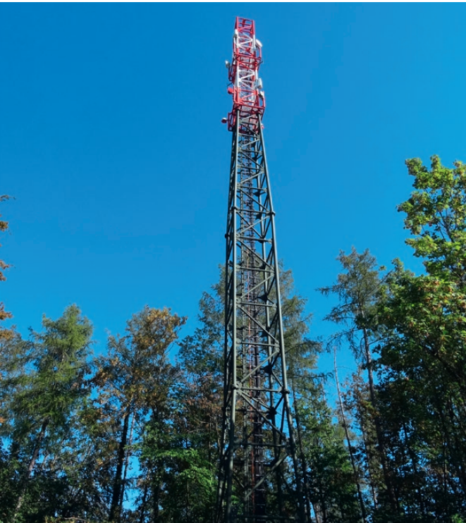
Funkmast in Lausen
